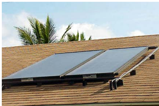
Flush mounted solar hot water panels
